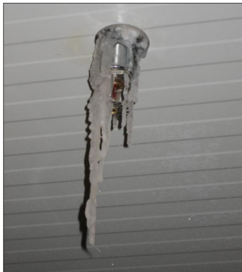
Kondensat in TK - Lager
